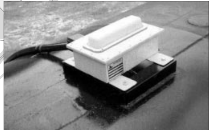
A typical installation on a tank car
