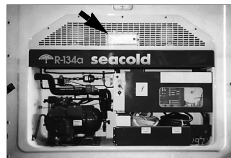
An example of CLR on a reefer container
